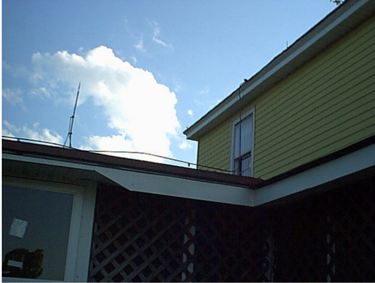
Figure 3. Detail of conductor installation showing improper conductor support. The conductor span between the upper and lower roof levels did not initially meet the support requirements of NFPA 780, 3-9.6. The support provided has become detached from the roof. Restraining the conductor is important since forces developed during a lightning event could cause it to fail. Environmental factors such as wind can also cause wear and ultimate failure in this case.
