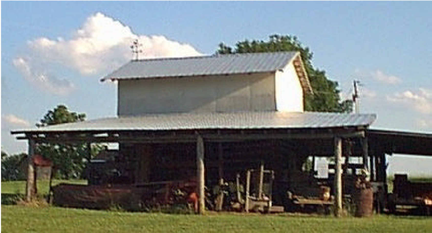
Figure 1. Barn with a decorative air terminal and no associated down conductors or grounding electrodes. If lightning attaches to this air terminal, it will seek a path through the structure. This would have the effect of blowing apart any moist wood or igniting dry wood. If lightning attaches to the thin metal roof, it will most likely cause burnthrough igniting combustible materials within the structure.
