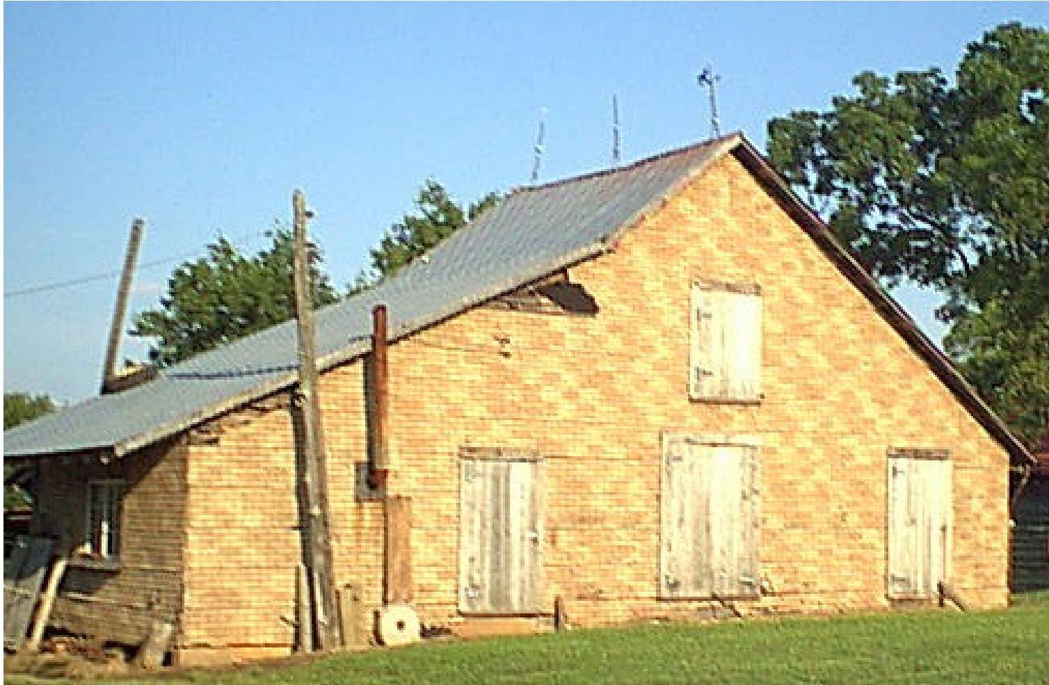
Figure 9. Example of leaning air terminals due to improper maintenance of air terminal support.
