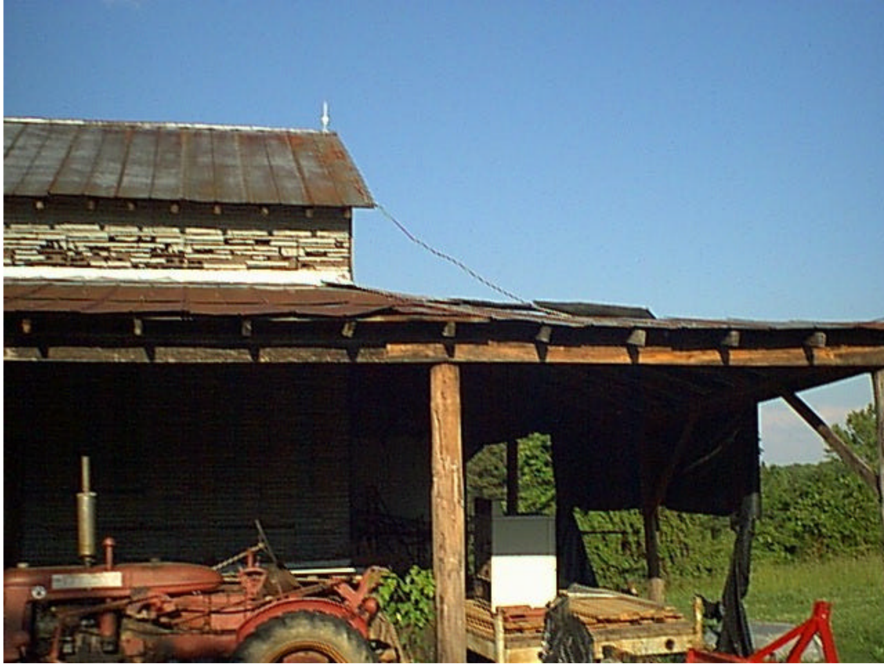
Figure 8. Example of improper conductor support due to lack of system maintenance.
