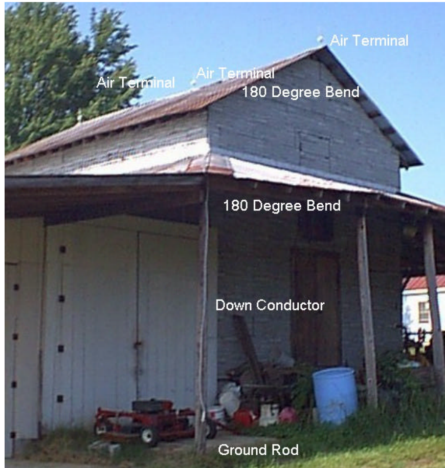
Figure 6. Example of lightning protection system on farm shop structure. Two 180 degree bends were formed in the northern down conductor. Testing and field experience reveals that this will fail during a lightning strike, causing a high temperature spark which could ignite the structure.
