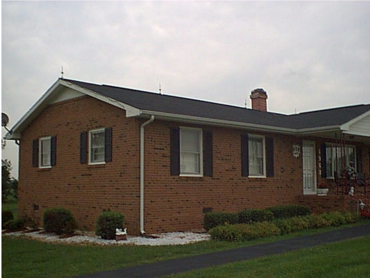
Figure 5. Example of residential installation where chimney was not provided with an air terminal. Also note the installation of Satellite Dish which is not protected by the initial design.
