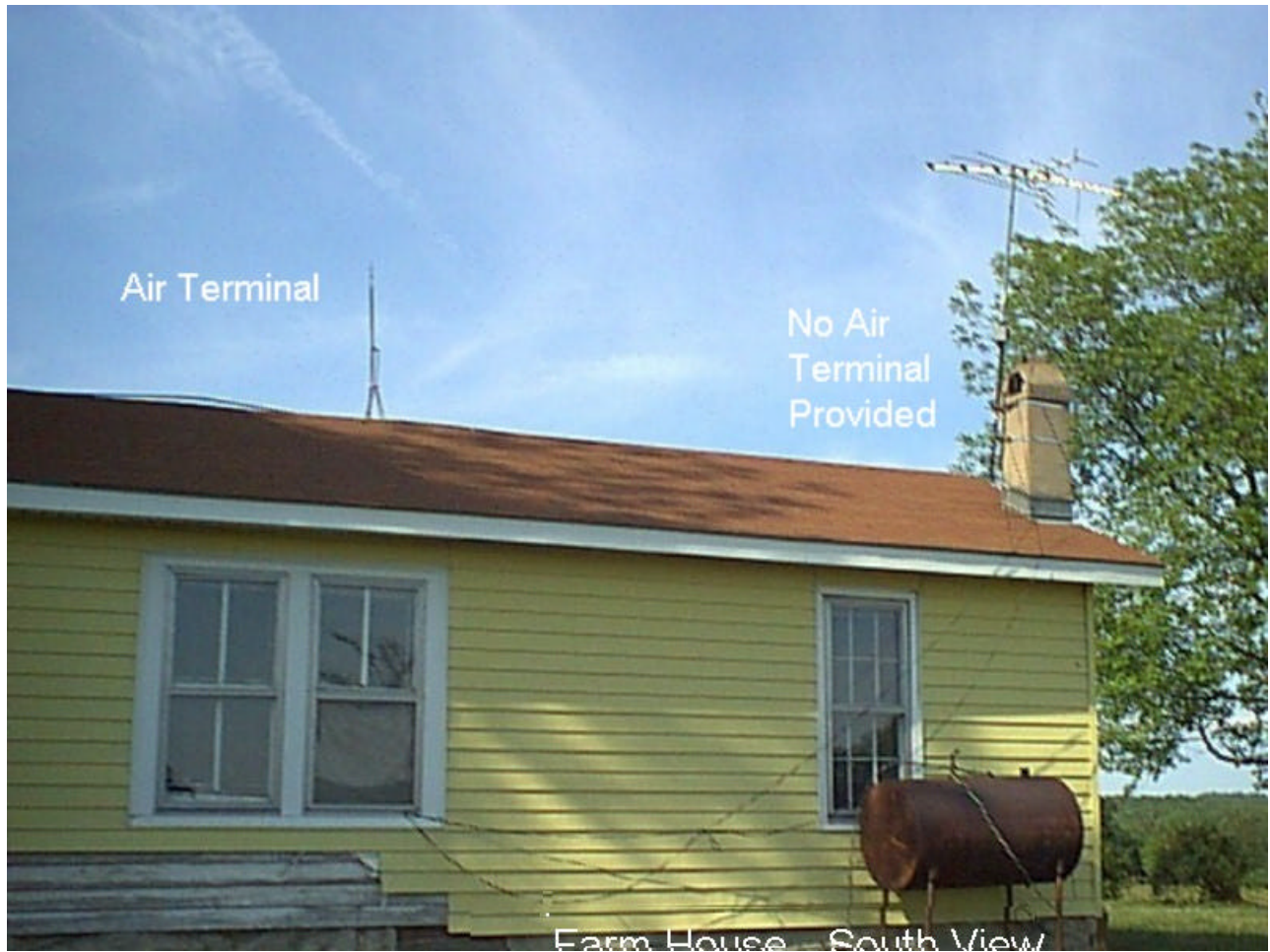
Figure 2. South View of Farm House lower level air terminal. Note there is no air terminal provided for the chimney and TV antenna. An attachment to either could prove very damaging. A lightning attachment to the chimney would likely cause it to fracture, while lightning to the antenna would likely be transferred to the structure of the house and enter through the lead in wire.
